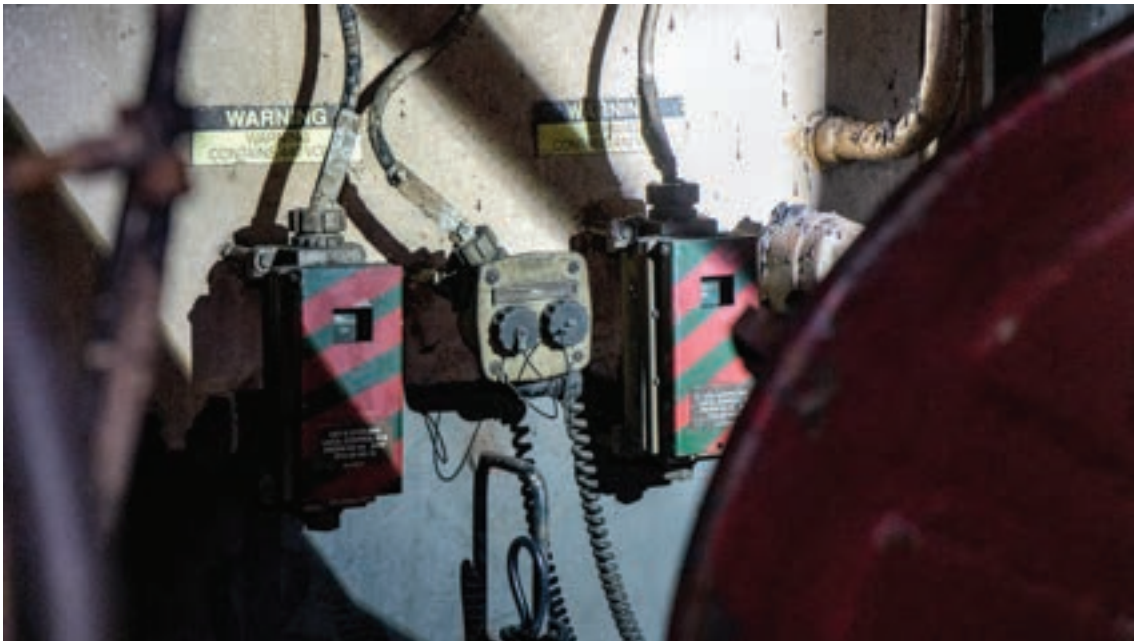
Figure 30, Still photo of AFFF push-buttons for sprinkler groups 15 and 16 serving Lower V with covers closed (16 on left; 15 on right). These push-buttons are in Upper V amidships. The photo shows proximity to open hatch, which obstructs visibility of the push
