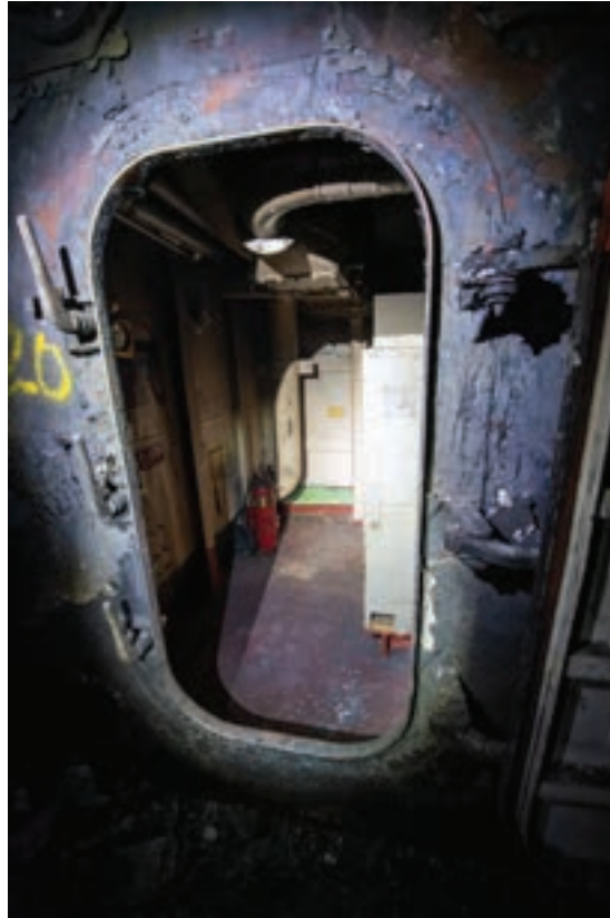
Figure 47 shows two compartments separated by a closed hatch. One compartment was severely damaged, while the adjacent compartment suffered minor damage.
