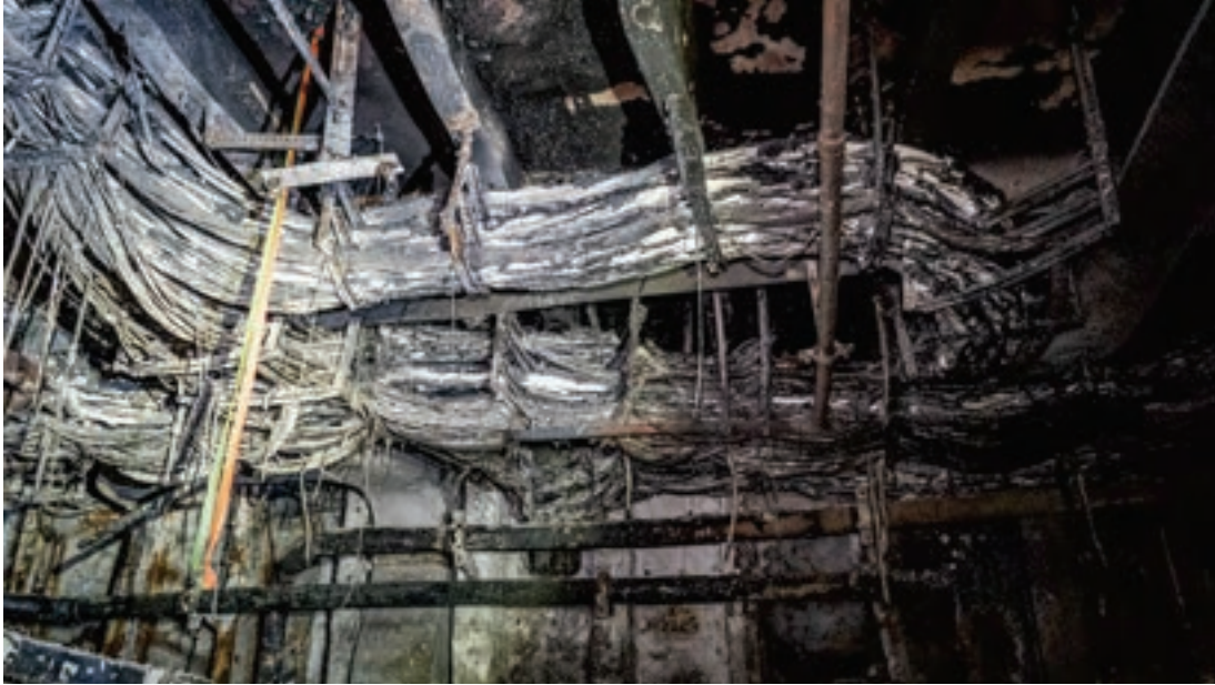
Figure 45 shows burned cableways in the Lower Vehicle Stowage Area (Lower V).
