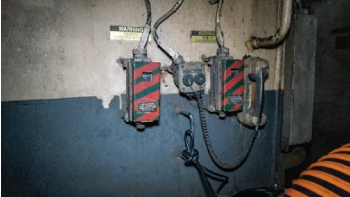
Figure 31, Still photo of AFFF push-buttons for sprinkler groups 15 and 16 serving Lower V with covers closed (16 on left; 15 on right). These push-buttons are in Upper V amidships.
